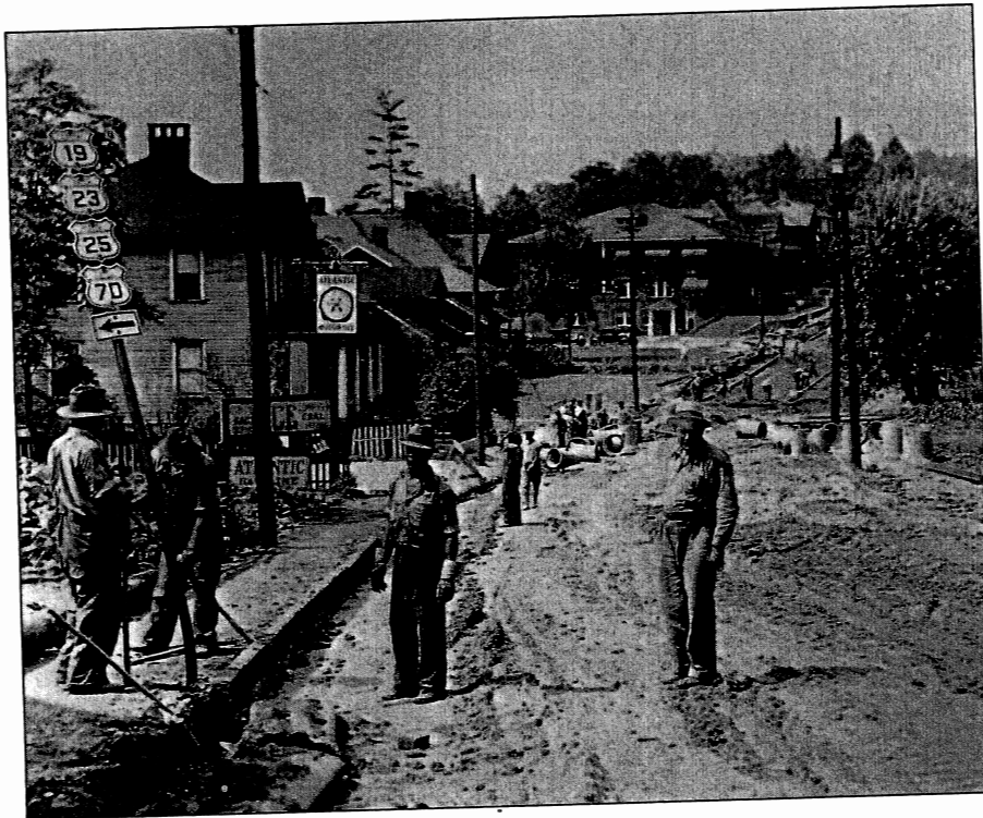
As part of a 1934 work relief project, FERA employees widened Merrimon Avenue in Asheville, North Carolina.
